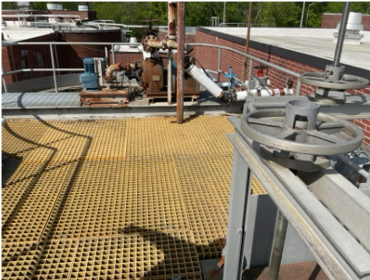
Grit tank top side
