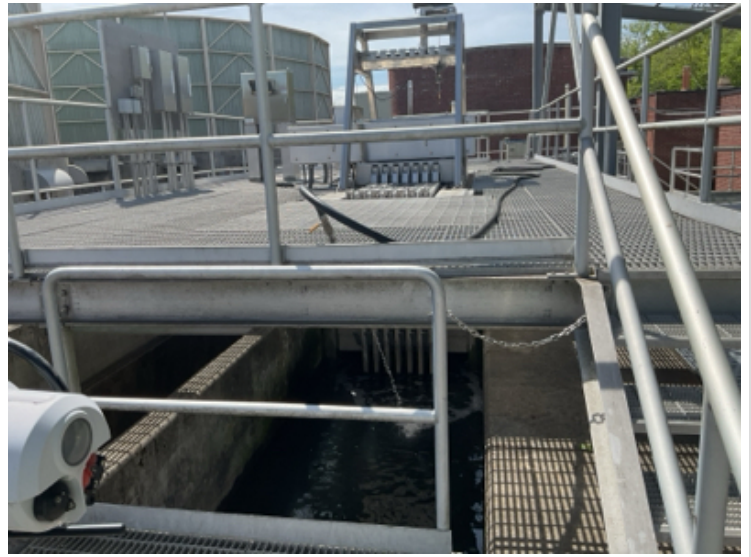
Existing UV unit
