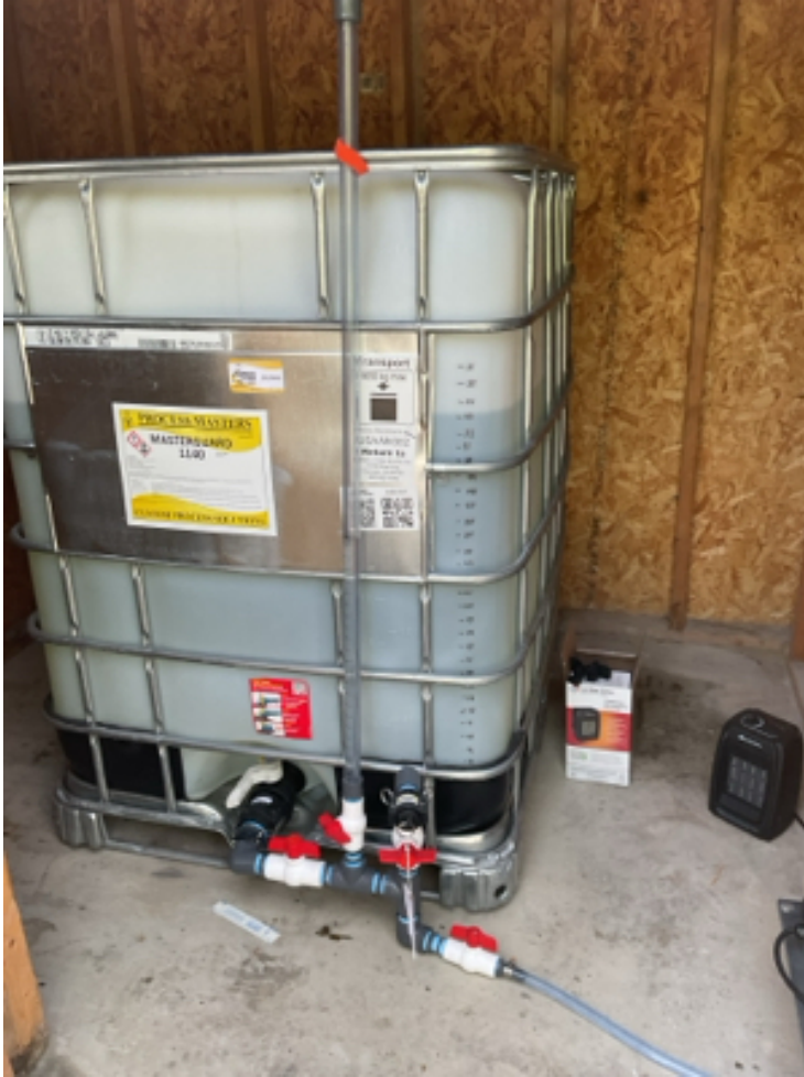
IBC tote in shed without containment
