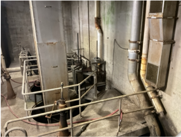
Head works metering and rag rakes
