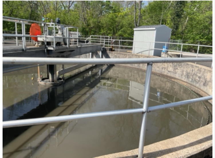
Thickener with shed holding an IBC tote for the pilot project.
