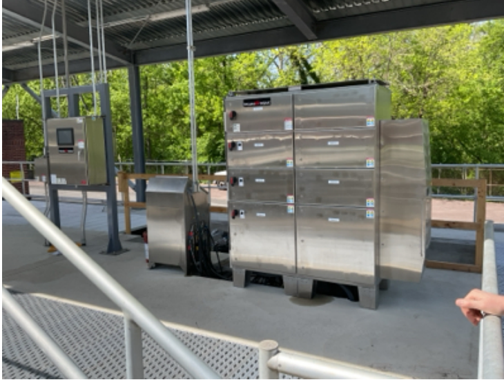
Newly installed UV unit
