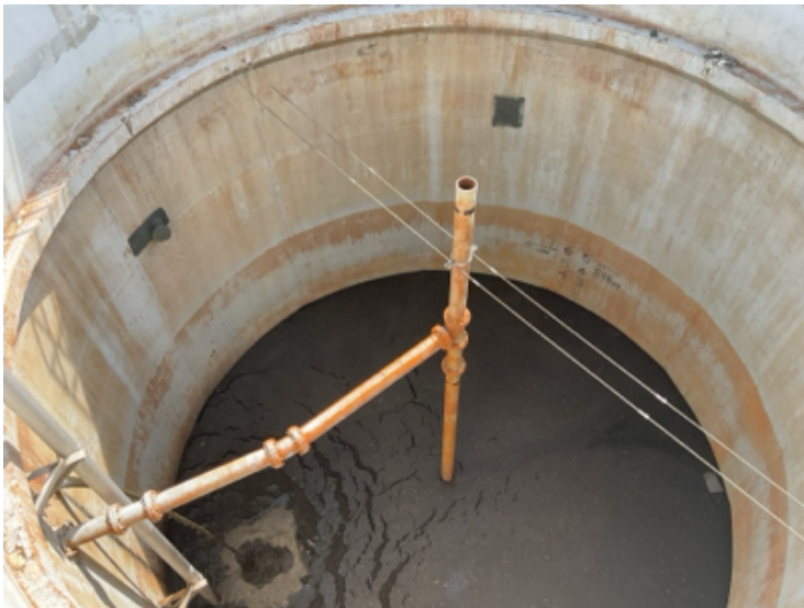
Aerobic digester with low inventory
