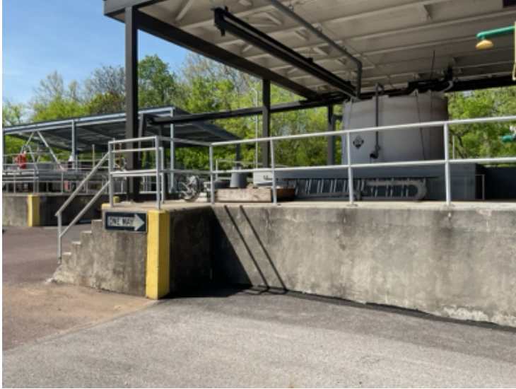
Hypochlorite tank in containment
