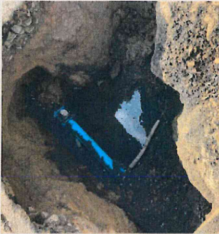
Francis Ave replaced section of 4" water main and portion of water service
