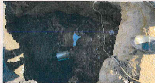
Edgewood Drive cracked main 6" main
